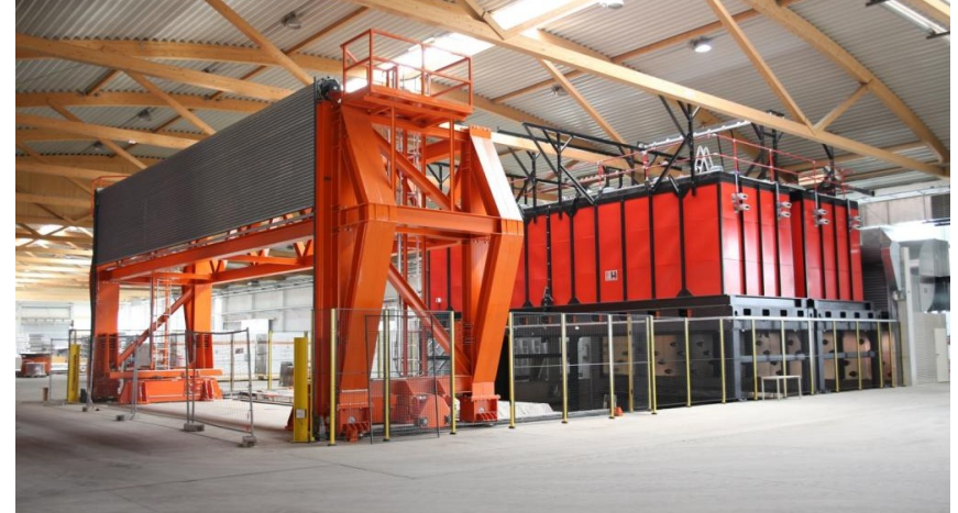
New hot ageing furnace and plate handling installed
